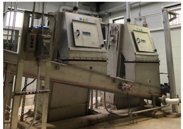
Automated screening machines remove any large debris that comes into the plant, to protect downstream equipment.
